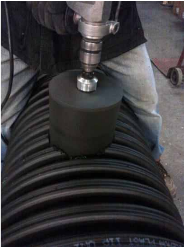
Drill the main pipe by using a drilling machine and milling cutter
